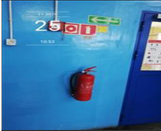
Photo of fire safety equipment IMG_20201125_105335.jpg
