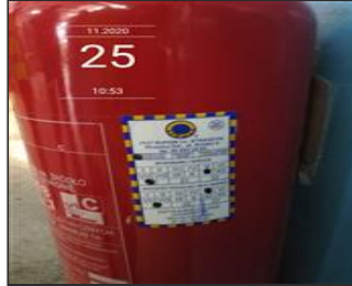
Photo of fire safety equipment IMG_20201125_105343.jpg
