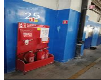
Photo of fire safety equipment IMG_20201125_110124.jpg
